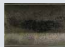
Eroded clamping section
